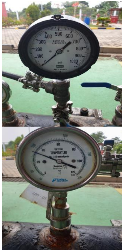
Gambar 5. Pressure dan Temperature Gauge
